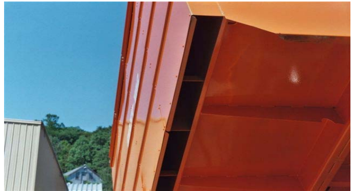
Downward Air Ducts for Leaf Chafe Exhaust - Down Draft
